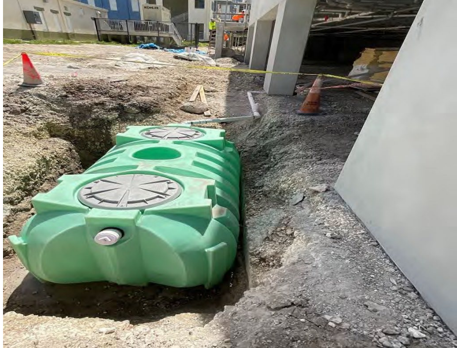
Sanitary Holding Tank
